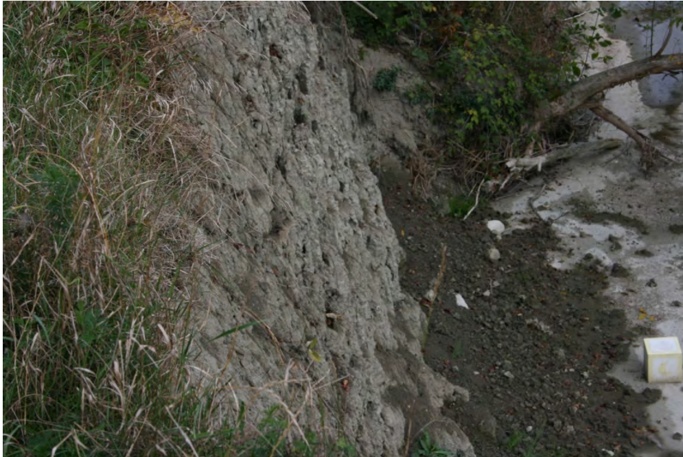
Photo Plate 3: View showing desiccation of the clay surface and bulk erosion collecting at the toe of the slope.
