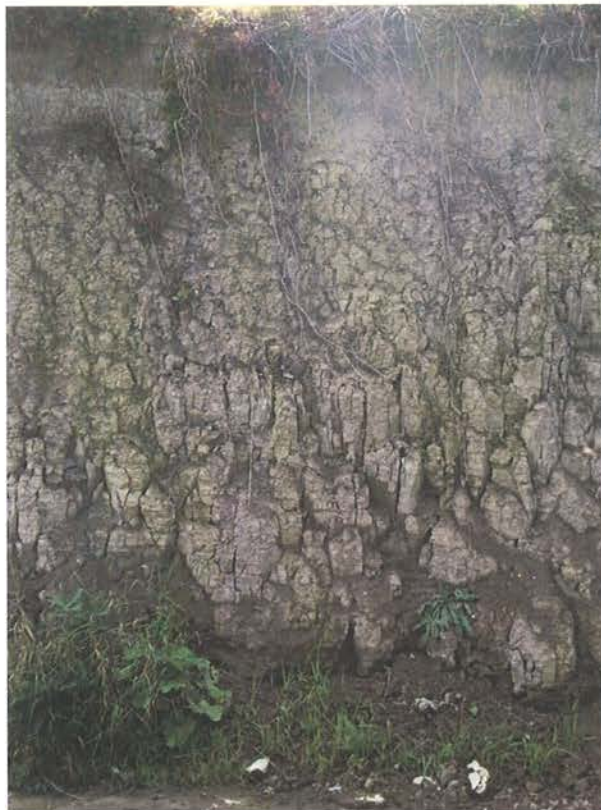
Photo No. 4: Desiccated and blocky clay on vertical slope face (west end).
