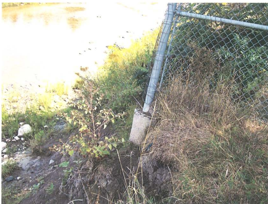
Photo No. 2: Exposed fence post foundation at east end of critical slope
