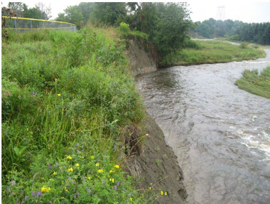
Photo Plate 1: View looking downstream at flow in contact with eroding bank under moderate flow conditions.
