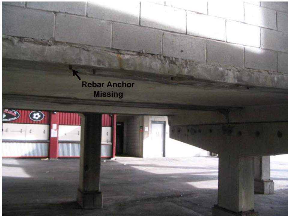
Photo 22 – Landing Ramp: Delamination slab edge; Guard rail anchors
