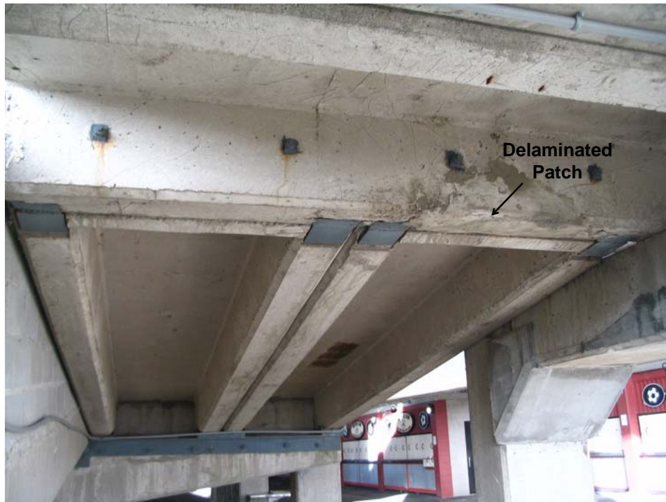
Photo 11 – Ramp R3 Hangers at R2: Delamination repair cracked
