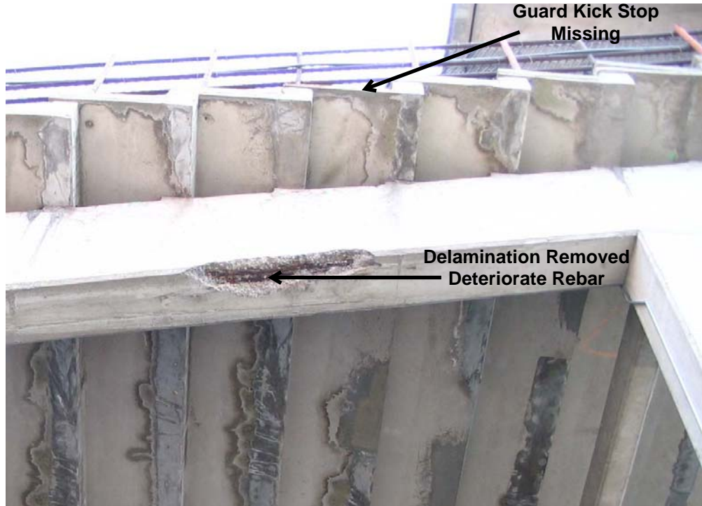
Photo 06 – Raker Beam 19: Deteriorated concrete/rebar; railing kick stop missing
