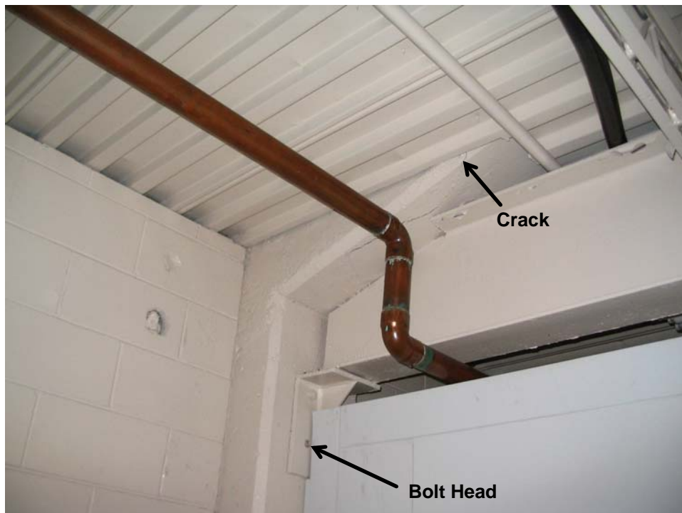
Photo 08 – Service building roof support at Frame 5: Bolt head removed; Raker Beam Cracks
