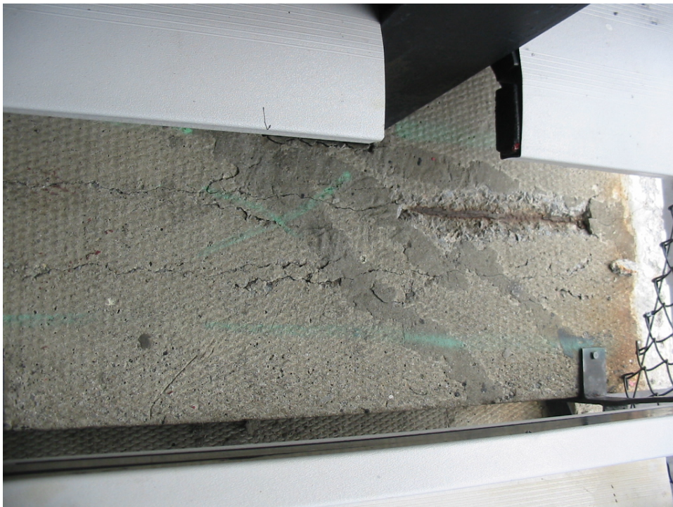
Photo 10 – Top of Precast Seating Panels: Deteriorated concrete and reinforcing
