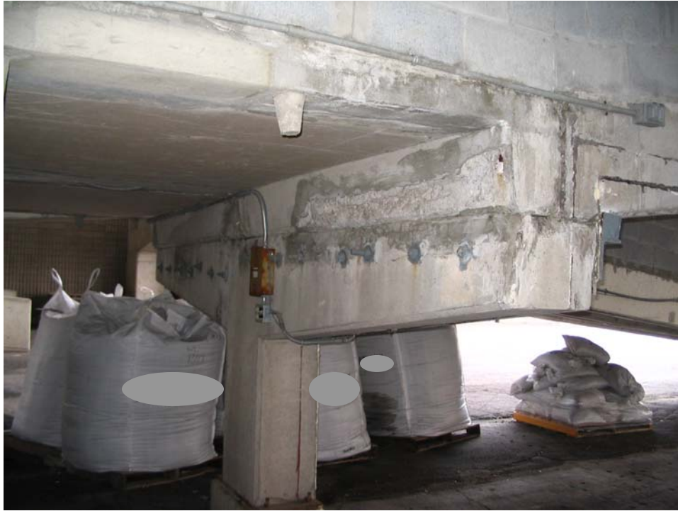
Photo 19 – Ramp Column Support @ Landing Slab: Guard rebar anchors; landing slab cracks; ramp column tee crack
