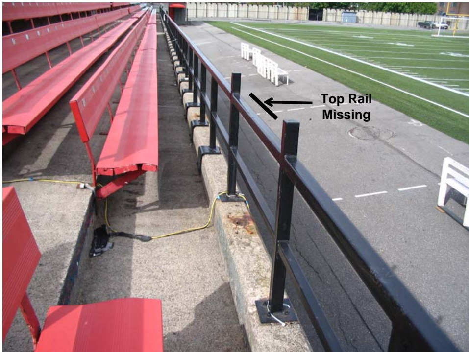
Photo 24 – Front aisle guard rail: Top horizontal rail missing
