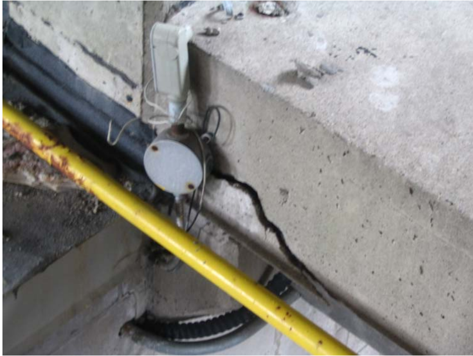
Photo 15 – Ramp Support Beam RB2: crack at support
