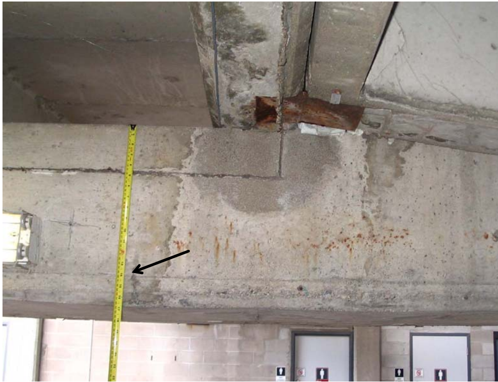
Photo 17 – Ramp Support Beam Cracks
