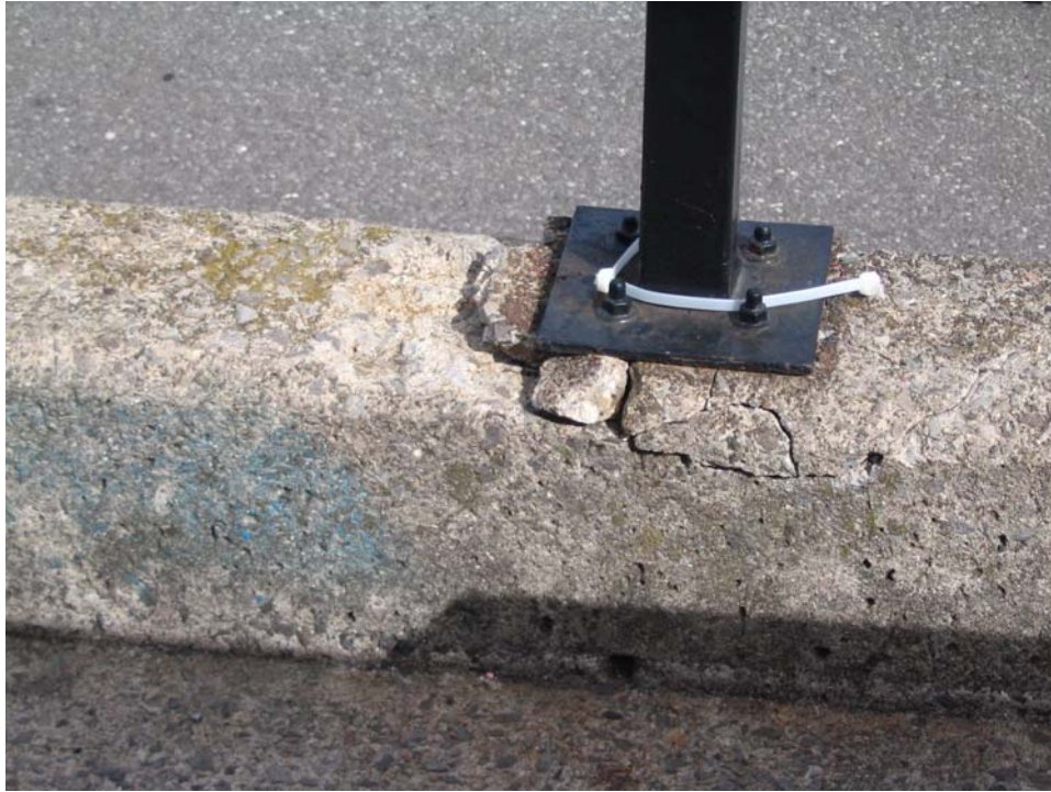
Photo 23 – Front Guard Rail: Deterioration base
