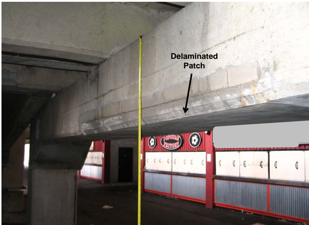
Photo 18 – Ramp Support Beam Delamination
