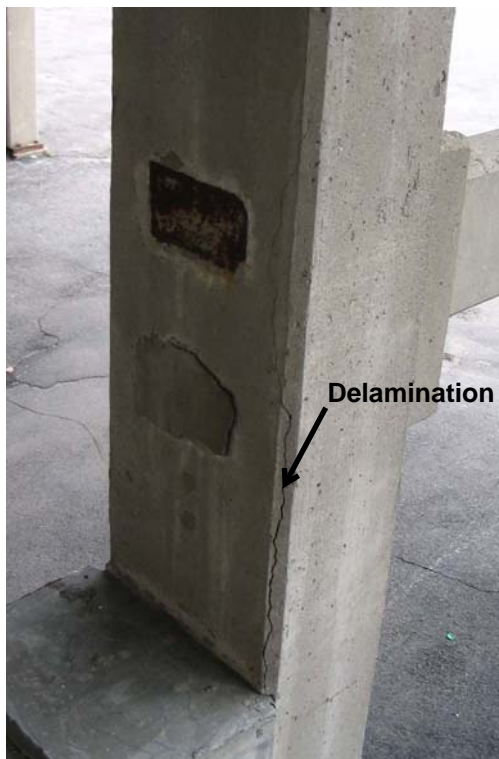
Photo 02 – Column C2: Local Deterioration
