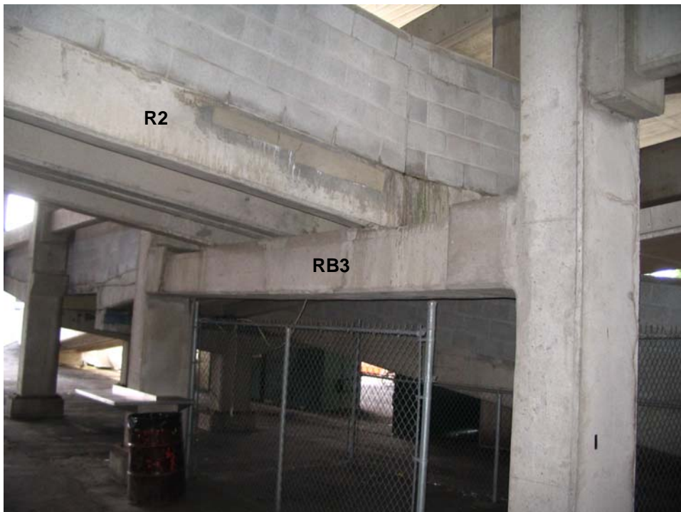
Photo 16 – Ramp Beam RB3: Deflection
