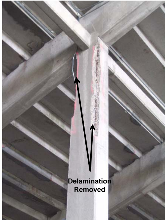
Photo 01 - Column @ Raker Beam: Concrete Spall
