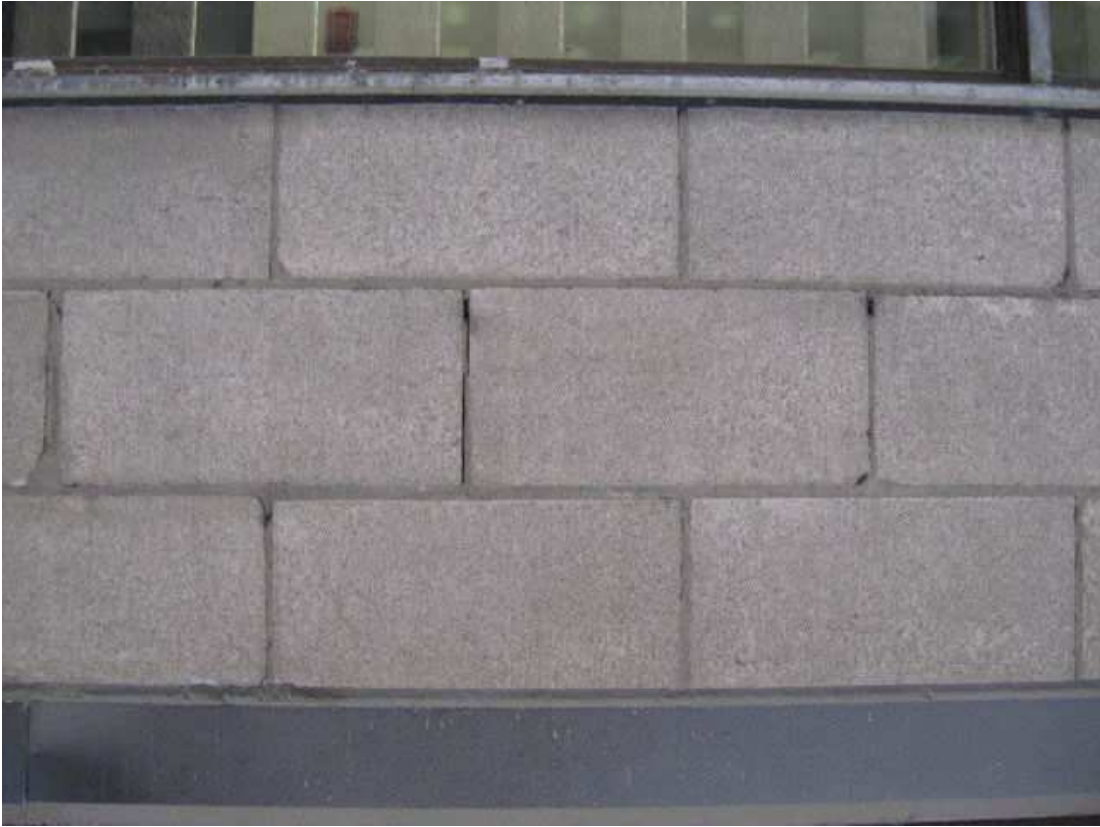
Photograph 9 - Deteriorated mortar at exterior block wall
