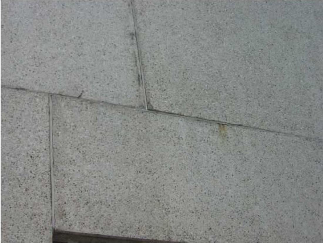
Photograph 15 - Chipped corner and corrosion staining
