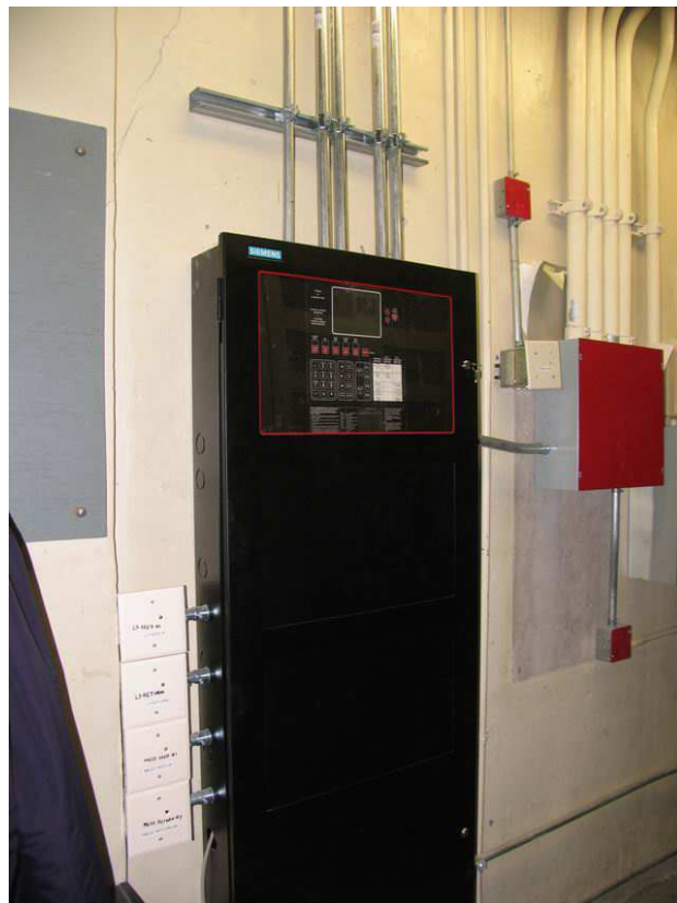
Photograph 40 - Main fire alarm panel
