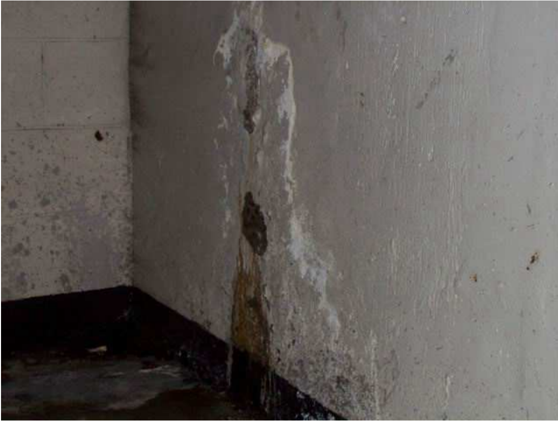
Photograph 5 - Wall cracking with corrosion staining
