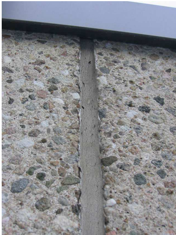
Photograph 22 - Alligator cracking of sealant
