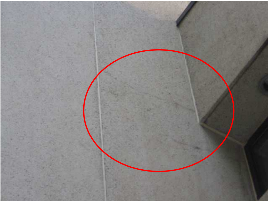
Photograph 10 - Cracking of precast panel
