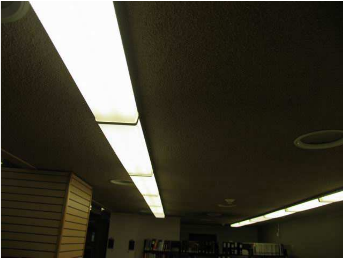
Photograph 43 - Surface mounted wrap around lens fixtures
