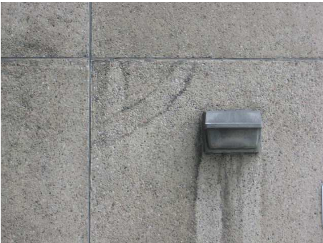
Photograph 12 - Staining of precast panel
