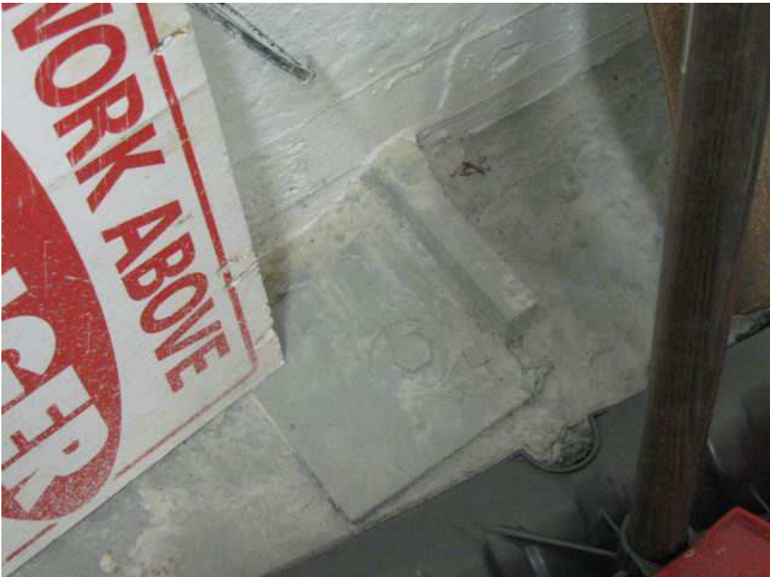
Photograph 20 - Misaligned connection with cast-in plate
