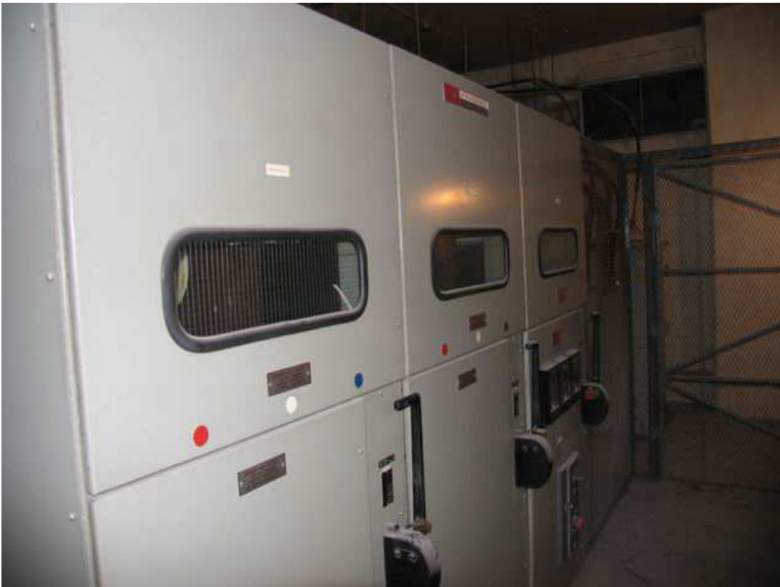
Photograph 30 - 15 kV switchboard in Hydro Vault
