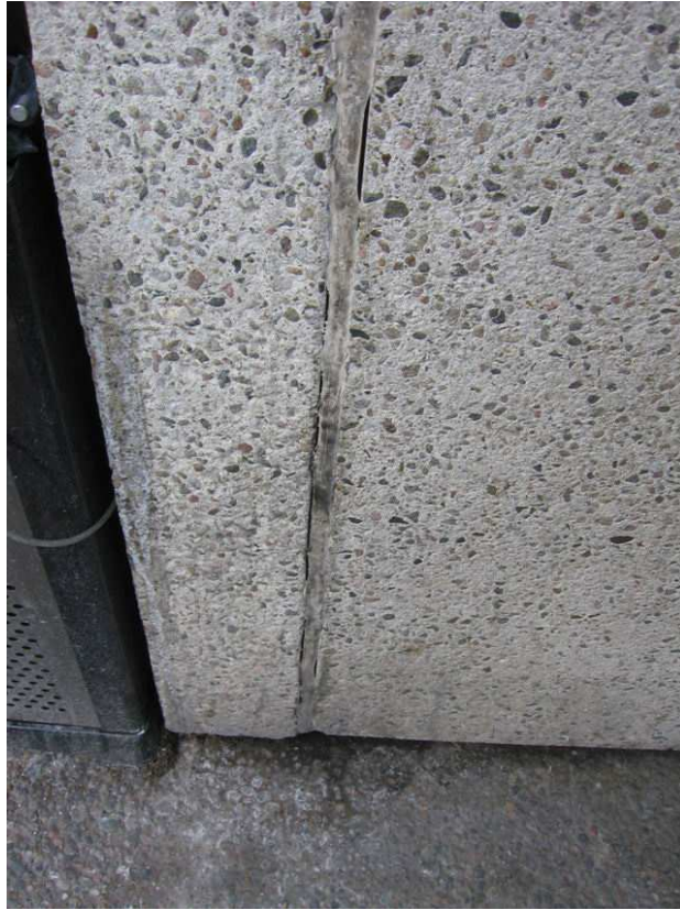
Photograph 23 - Sealant adhesive failure
