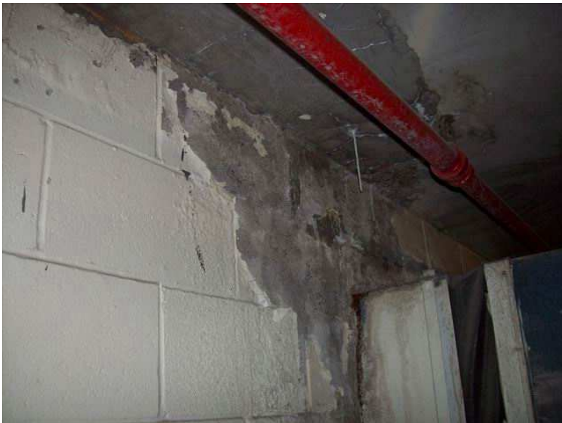
Photograph 4 - Concrete wall damage
