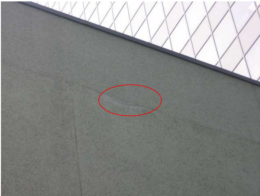
Photograph 18 - Crack in precast panel
