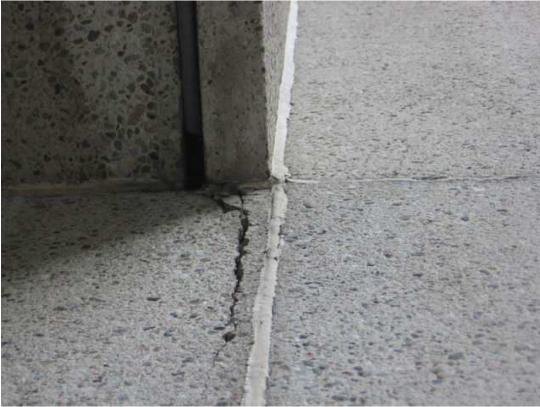
Photograph 13 - Cracked panel at grid line H
