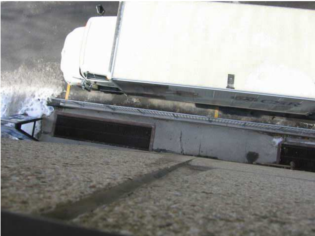
Photograph 16 - Crack in precast panel
