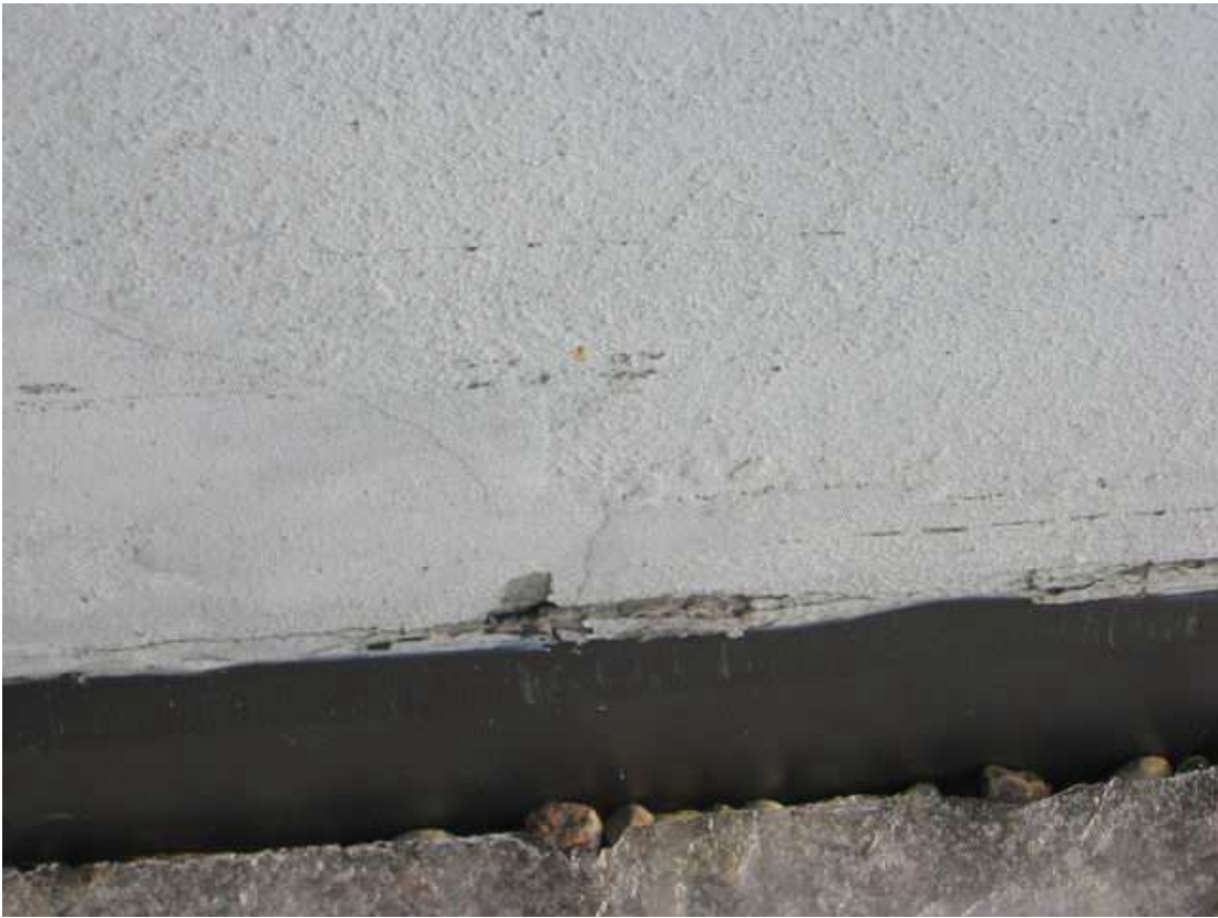
Photograph 27 - Damaged parking at parapet wall
