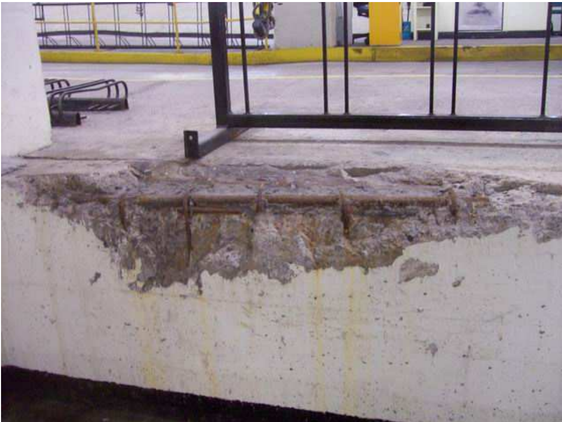
Photograph 6 - Spalled concrete at half wall
