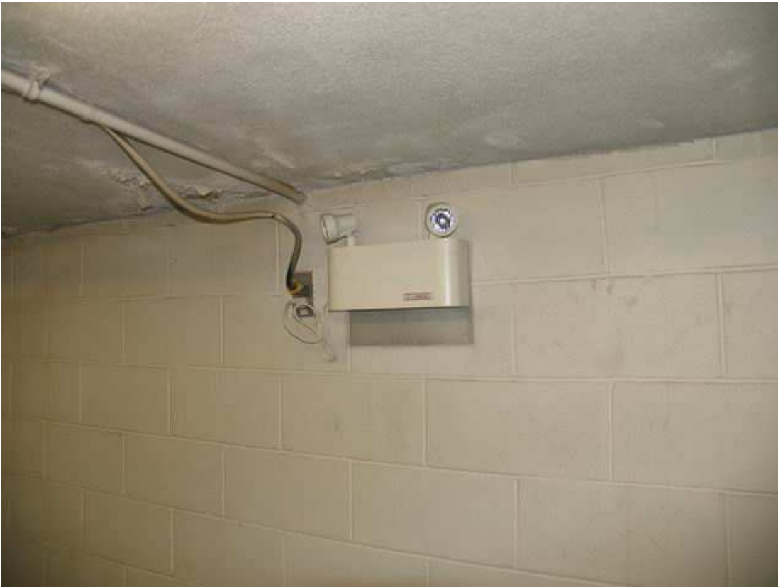
Photograph 45 - Emergency battery unit
