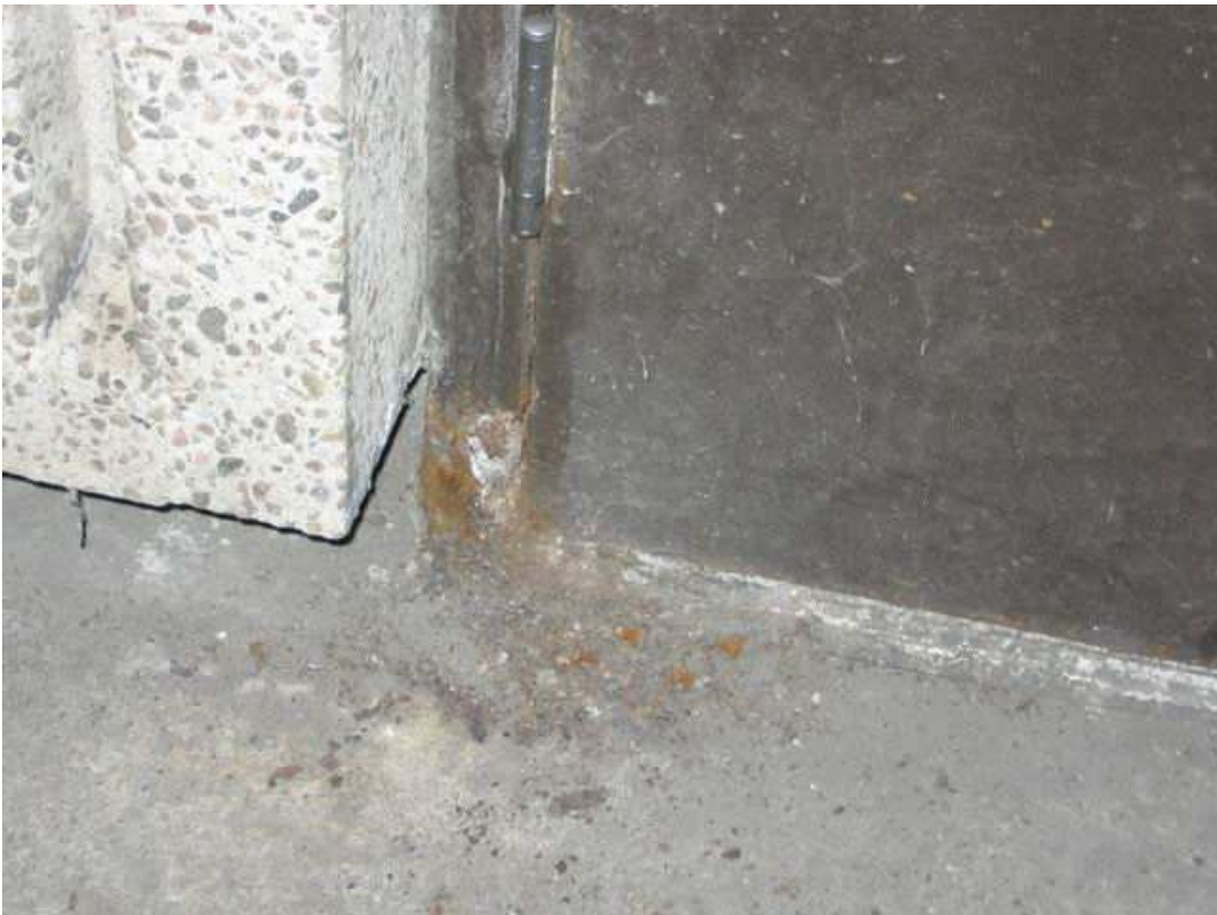
Photograph 26 - Corrosion of exterior door frame
