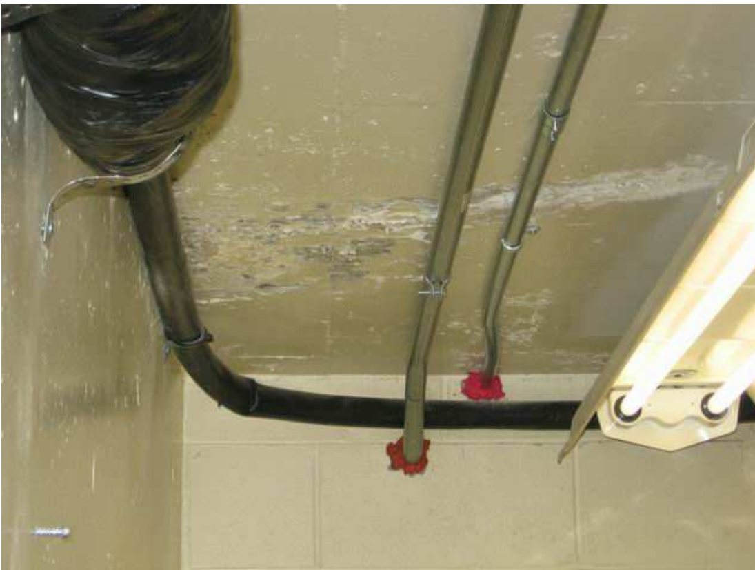
Photograph 8 - Water damage in server room
