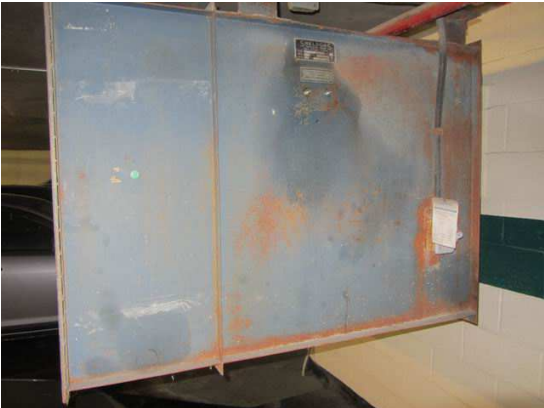
Photograph 48 - Corrosion of parking garage exhaust fans
