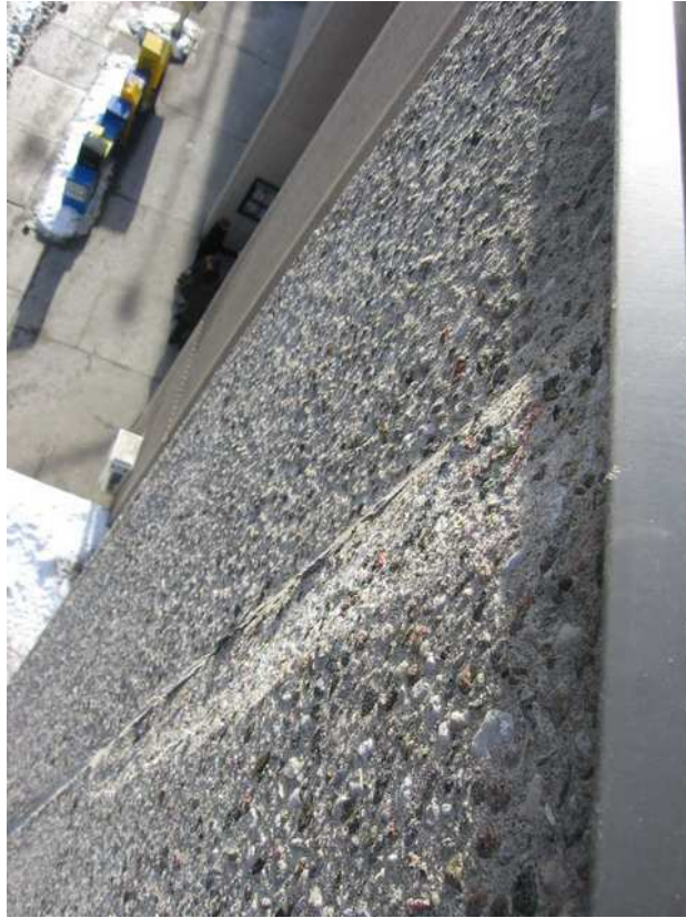
Photograph 17 - Scale on precast panel
