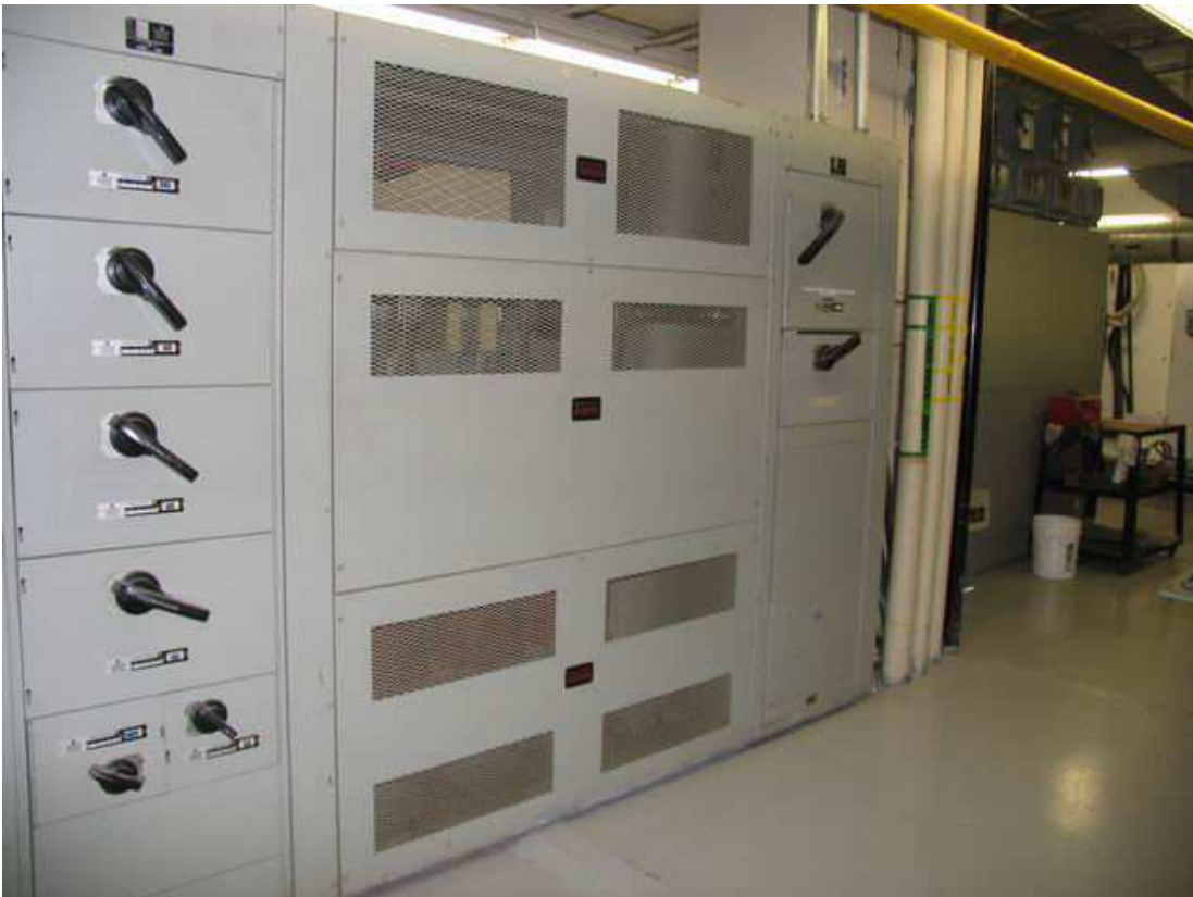
Photograph 34 - Penthouse Mechanical room switchboard
