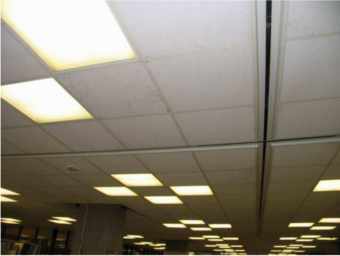
Photograph 41 - Lay-in fluorescent fixtures
