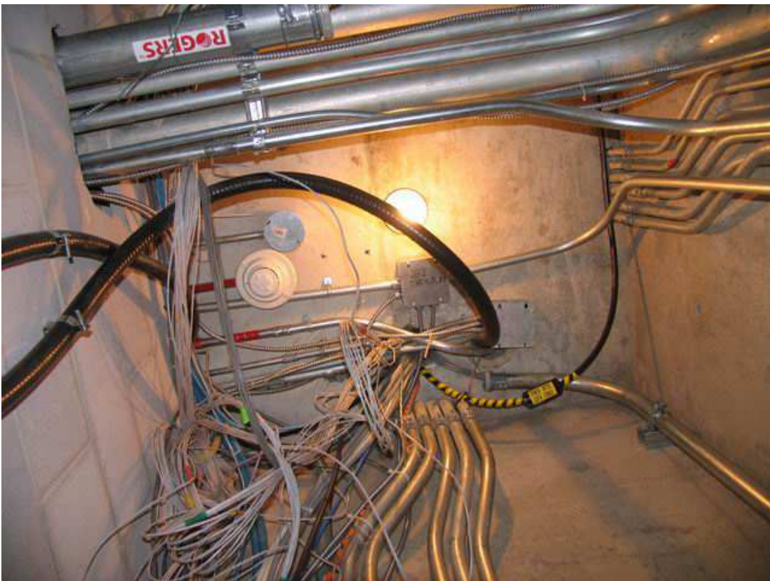
Photograph 46 - Typical data conductor installation
