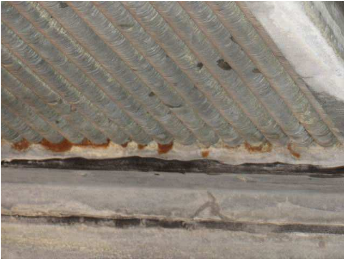
Photograph 47 - Tube end corrosion on cooling coil
