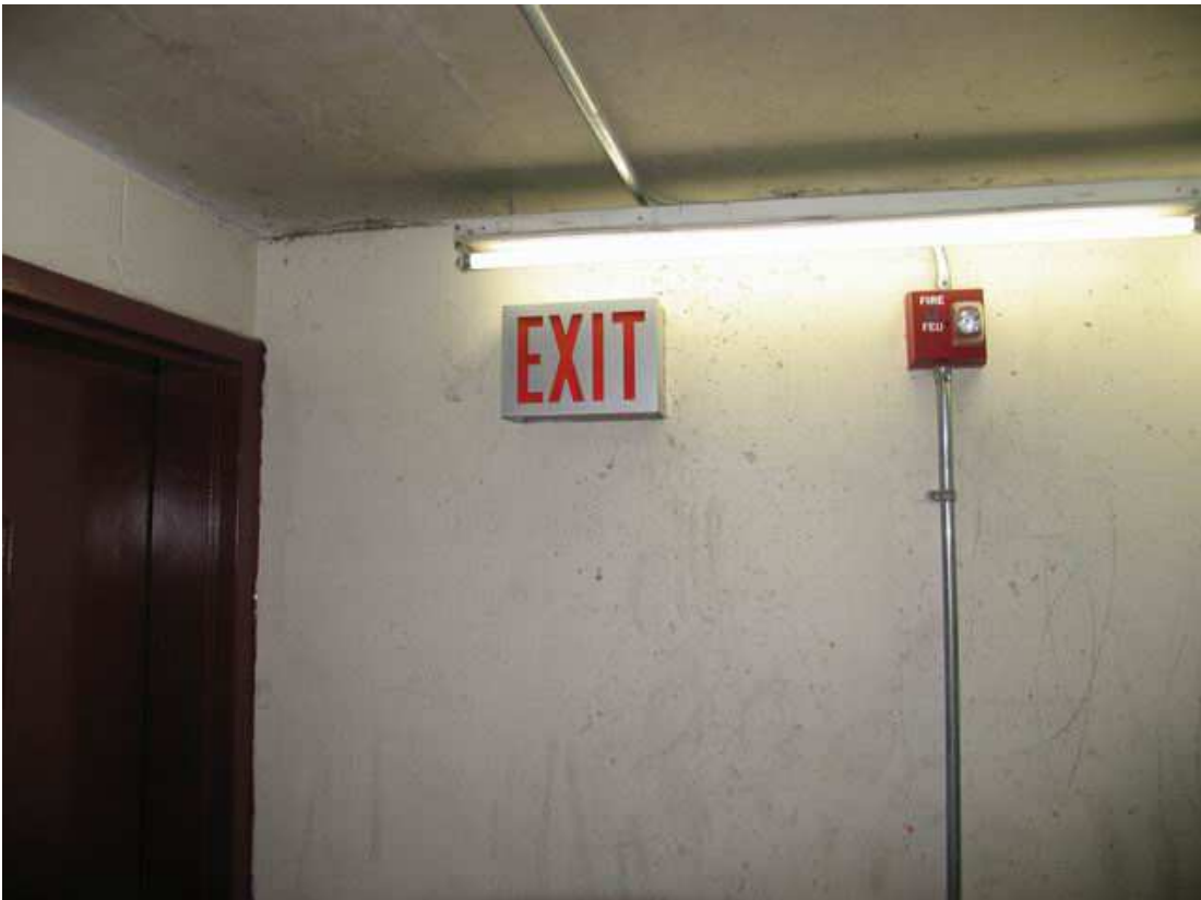
Photograph 44 - Typical exit sign
