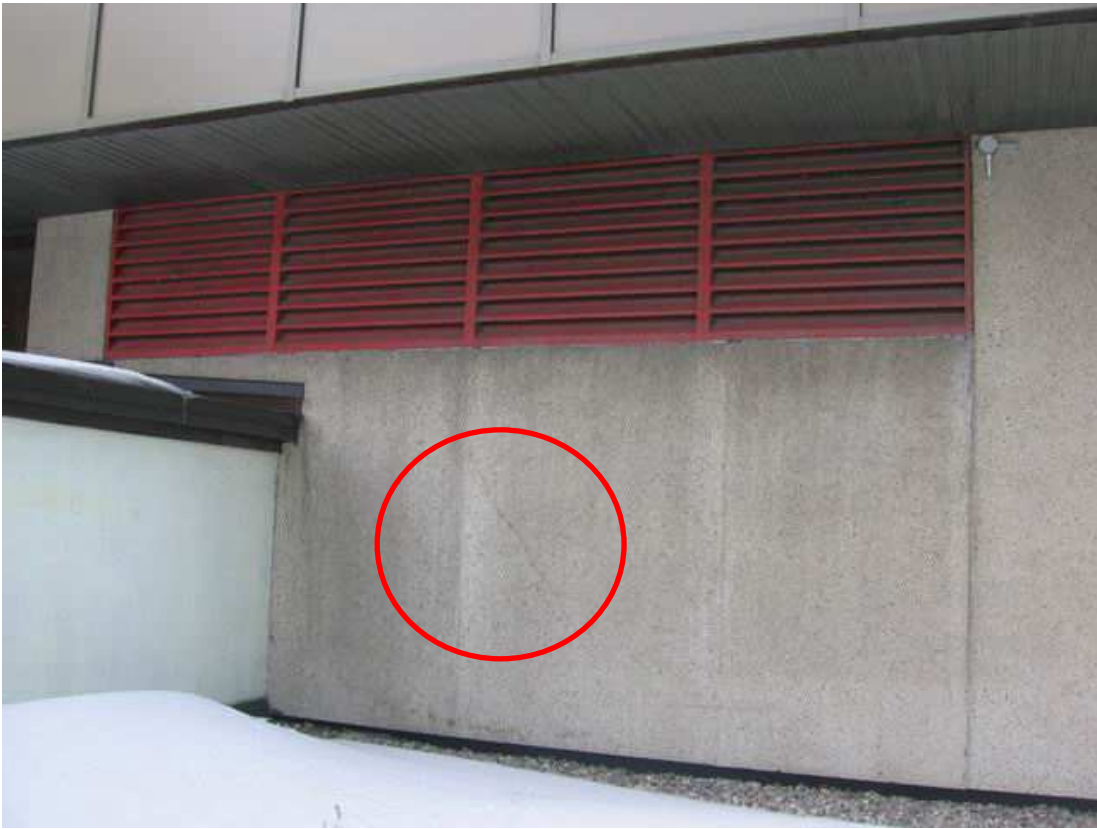
Photograph 11 - Cracking of precast panel
