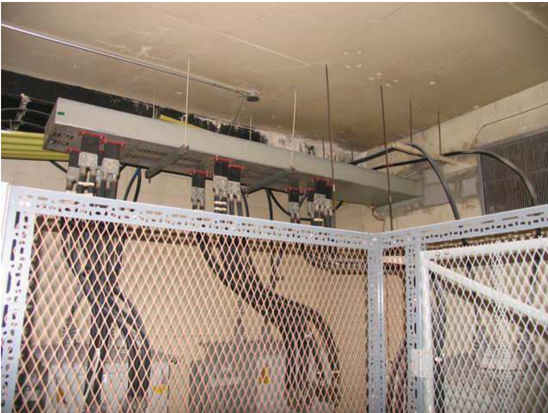
Photograph 32 - Bus duct and drip shields
