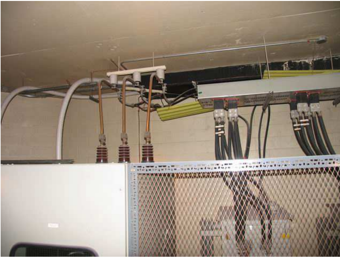
Photograph 31 - IPS bus and bus duct
