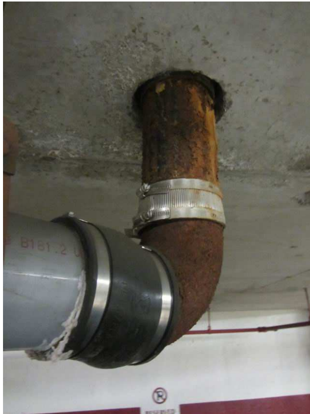
Photograph 49 - Corrosion of drainage piping in the parking garage
