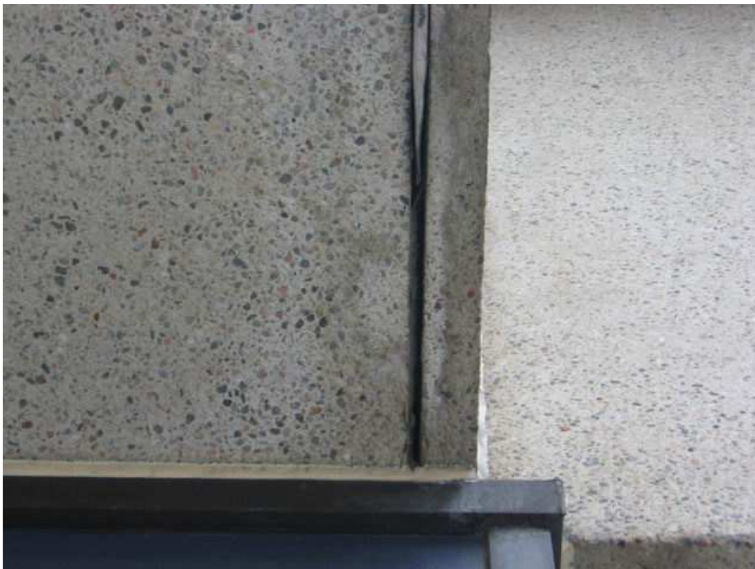
Photograph 24 - Missing sealant at soffit
