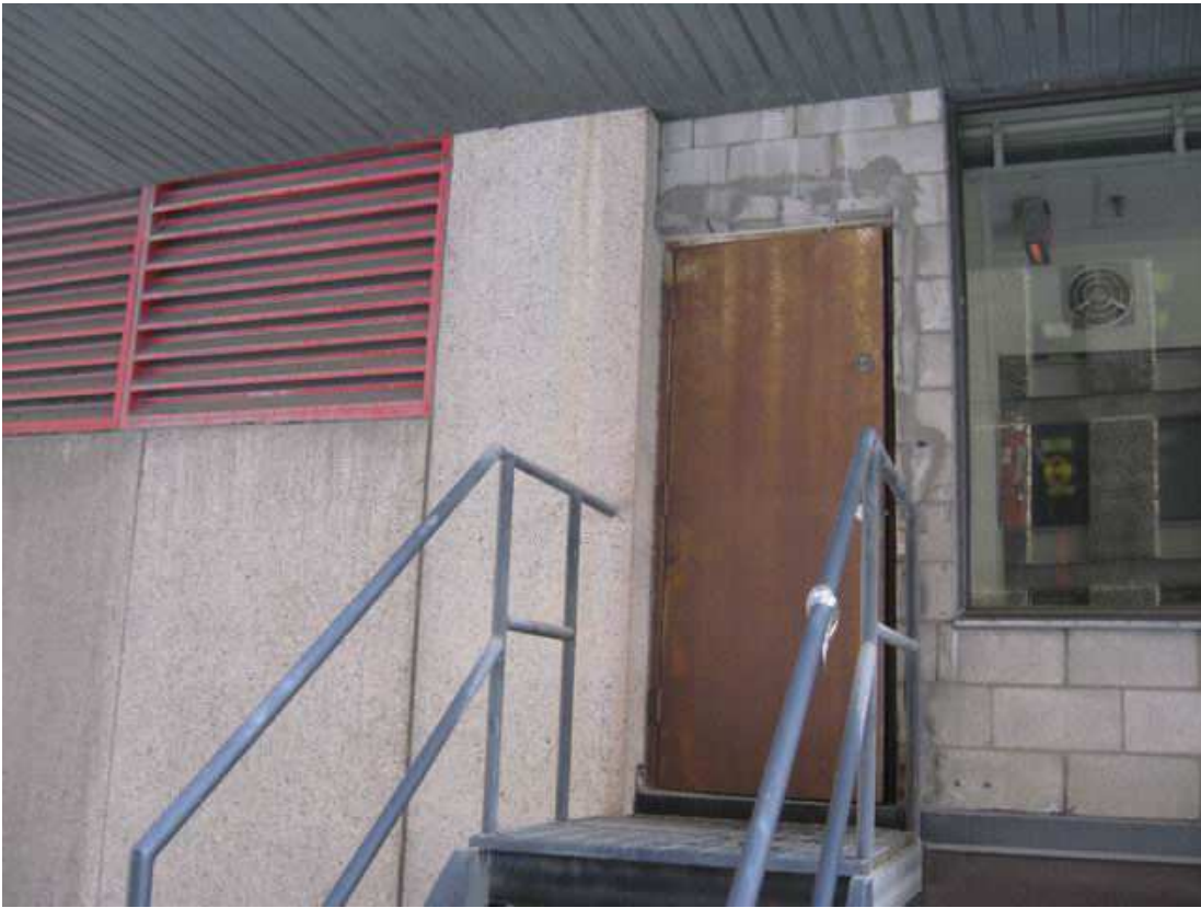
Photograph 25 - Corrosion of roof access door
