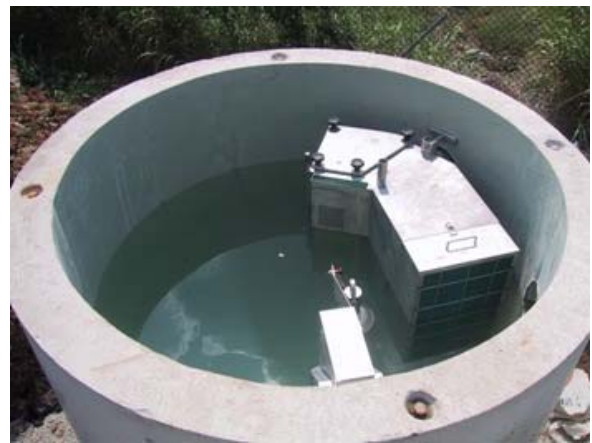
Figure 10: Oil and Grit Separator 19
